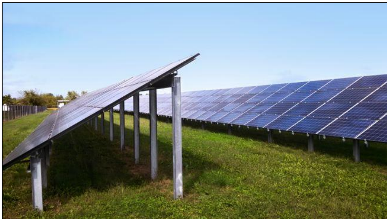
Figur 4. Fixed-tilt-anlegg / anlegg med faste stativer (foto: Willowbrook Solar Farm ( https://www.willowbrooksolar.com/resources )).
